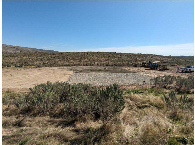
Figure 3. Groundwork progress for the construction of the carcass disposal station. Next, contractors will lay an asphalt pad.
